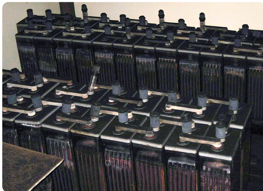
Lead-acid battery bank: cheap and proven — but only 50 % of the capacity usable (photo: Pseudoznanstvenik, CC BY-SA 3.0, via Wikimedia Commons)
